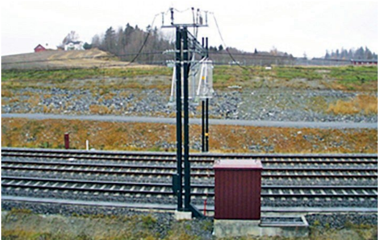
Figur 18.2 Sugetransformator plassert i kiosk
